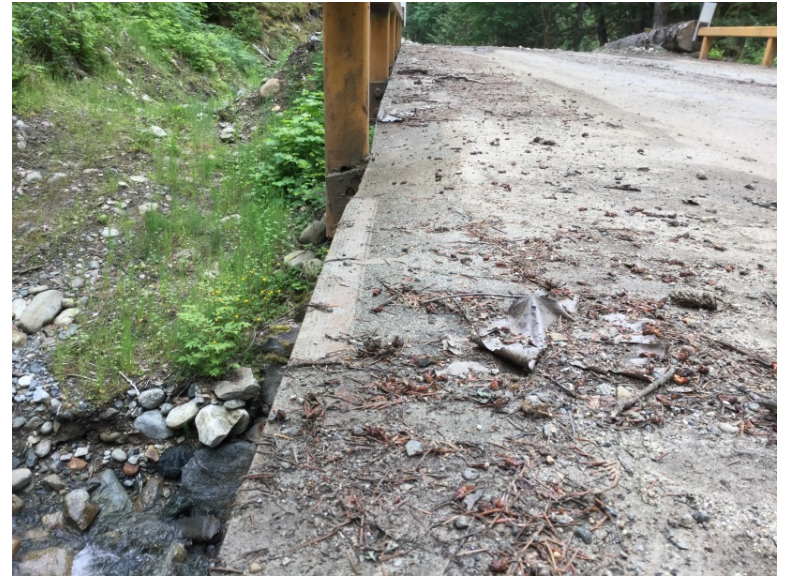
Damage noted to outside deck edge on upstream box girder
