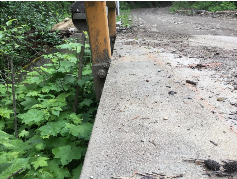
Damage noted to outside deck edge on downstream box girder
