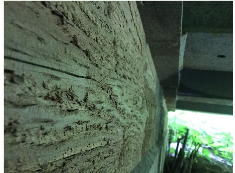
Bearing plate not completely on sill at right bank, up to 100mm off
