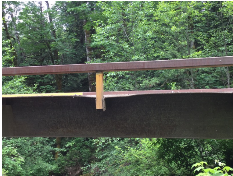
Damage to upstream box girder
